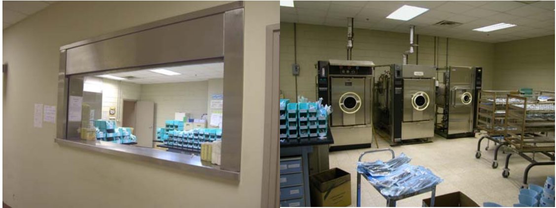
Figure.2: Photographs showing the: a. A CSSD Window for handling instruments to students, b. The main CSSD
